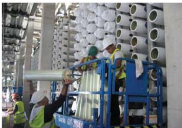
Hadera desalination plant
