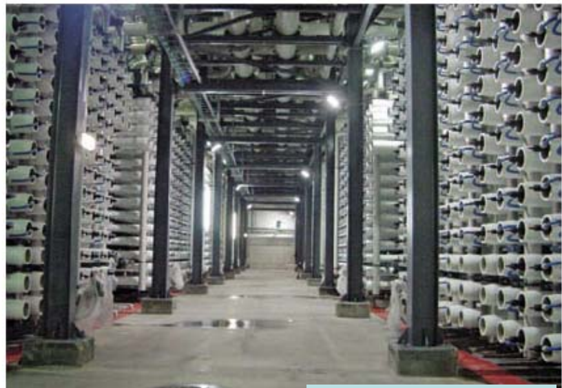
Ashkelon desalination plant
